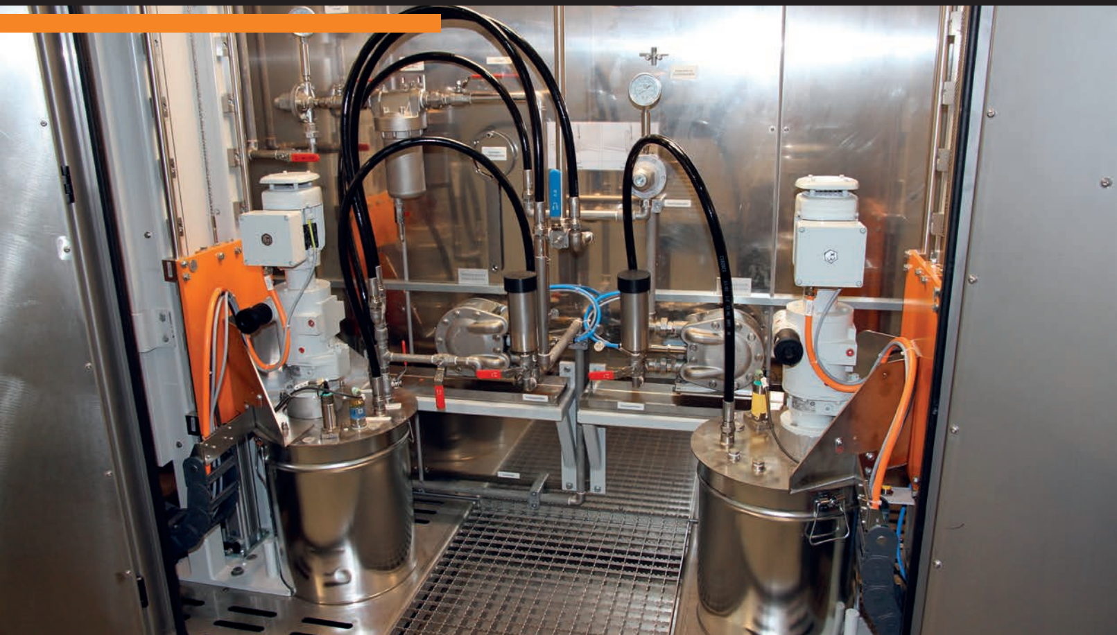
Typical paint supply for small containers (30 kg standard hobbocks) incl. automat. refill container, explosion protected design
